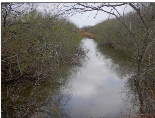
Photograph 3 – View looking east at the existing Delta Lake Drain from Private Culvert Crossing #1.
