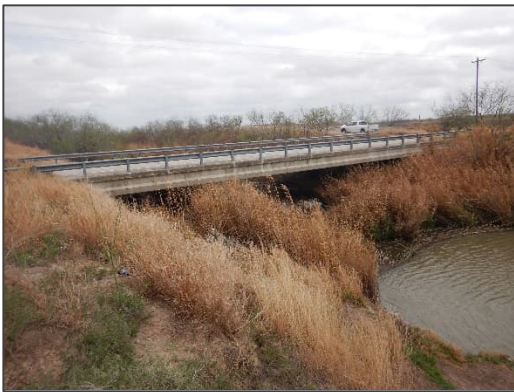
Photograph 38 – View looking northeast at the existing Delta Lake Drain as it flows under County Road (CR) 2900 West.
