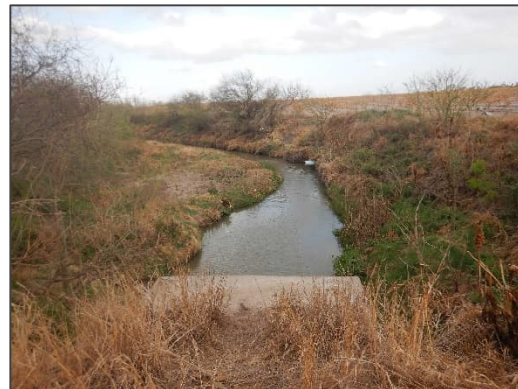
Photograph 23 – View looking east (downstream) at the existing Delta Lake Drain from Mile 5 1/2 West Road.
