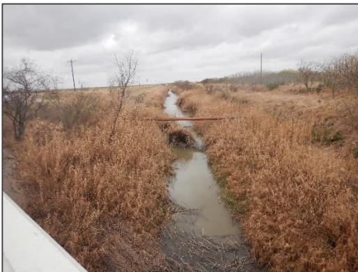
Photograph 33 – View looking southwest (upstream) at the existing Delta Lake Drain from the FM 1015 bridge.
