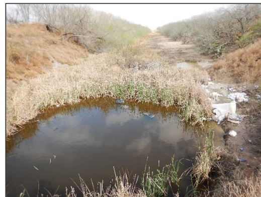
Photograph 5 – View looking east (downstream) at the existing Delta Lake Drain from FM 3444.
