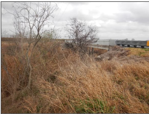
Photograph 32 – View looking northeast at FM 1015 as it crosses over the existing Delta Lake Drain.
