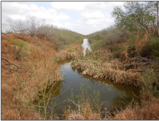
Photograph 7 – View looking east (downstream) at the existing Delta Lake Drain from Private Culvert Crossing #2.
