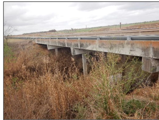
Photograph 35 – View looking northeast at the existing Delta Lake Drain as it flows under the FM 490 bridge.
