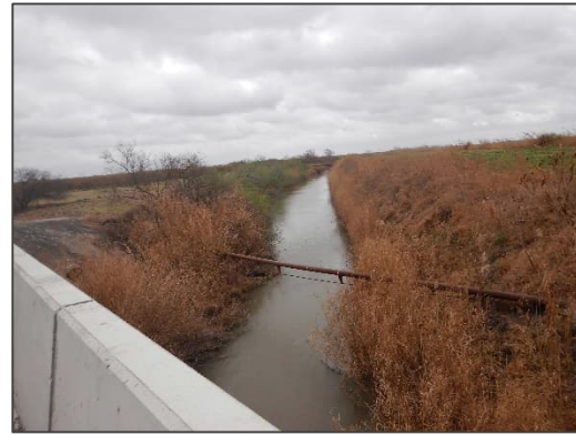
Photograph 34 – View looking northeast (downstream) at the existing Delta Lake Drain from the FM 1015 bridge.
